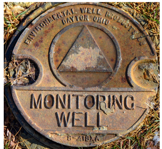
Groundwater Monitoring Well
